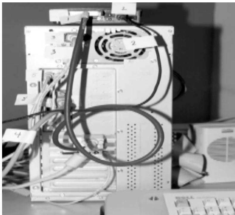
Figure 5 – Using Labels to Number Cables and Corresponding Ports
